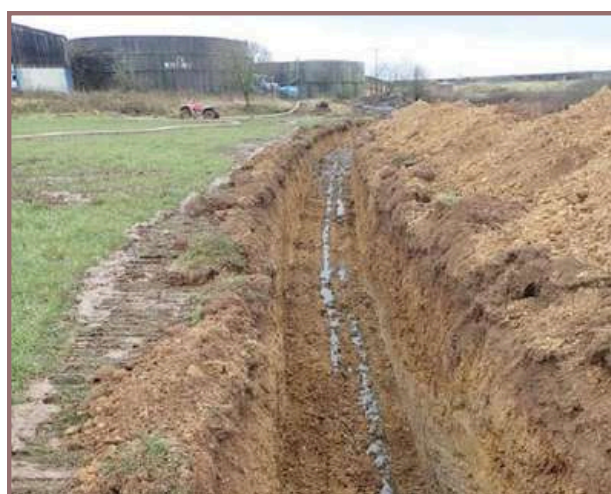
Slurry interception ditch © NDPA
