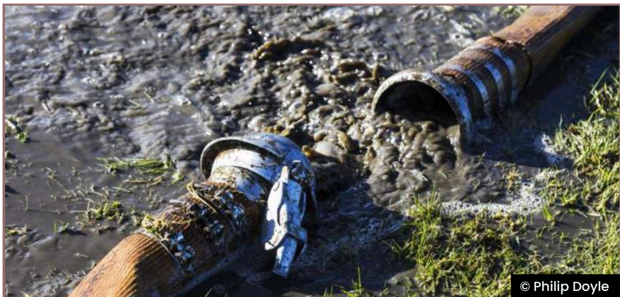
Broken slurry pipe © Philip Doyle
